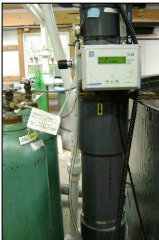
Water monitoring system and oxygenation tanks
