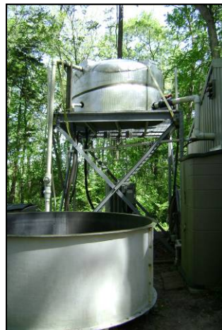
1,200 gallon elevated water tank
